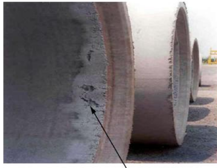
Figure 12—Repairable Honeycombing (Photo Courtesy of ACPA)
