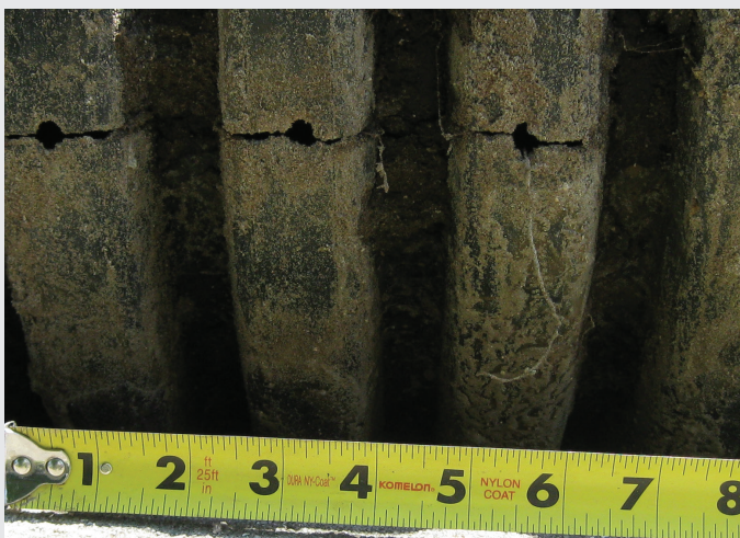
This HDPE pipe was deflected and cracked at the springline, passing through the ~1/8-inch holes that had been drilled into each corrugation.
