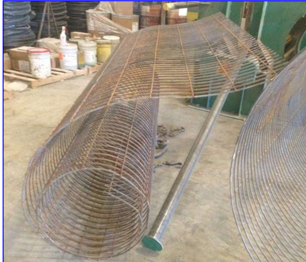
Improper Cage Machine Set Up
