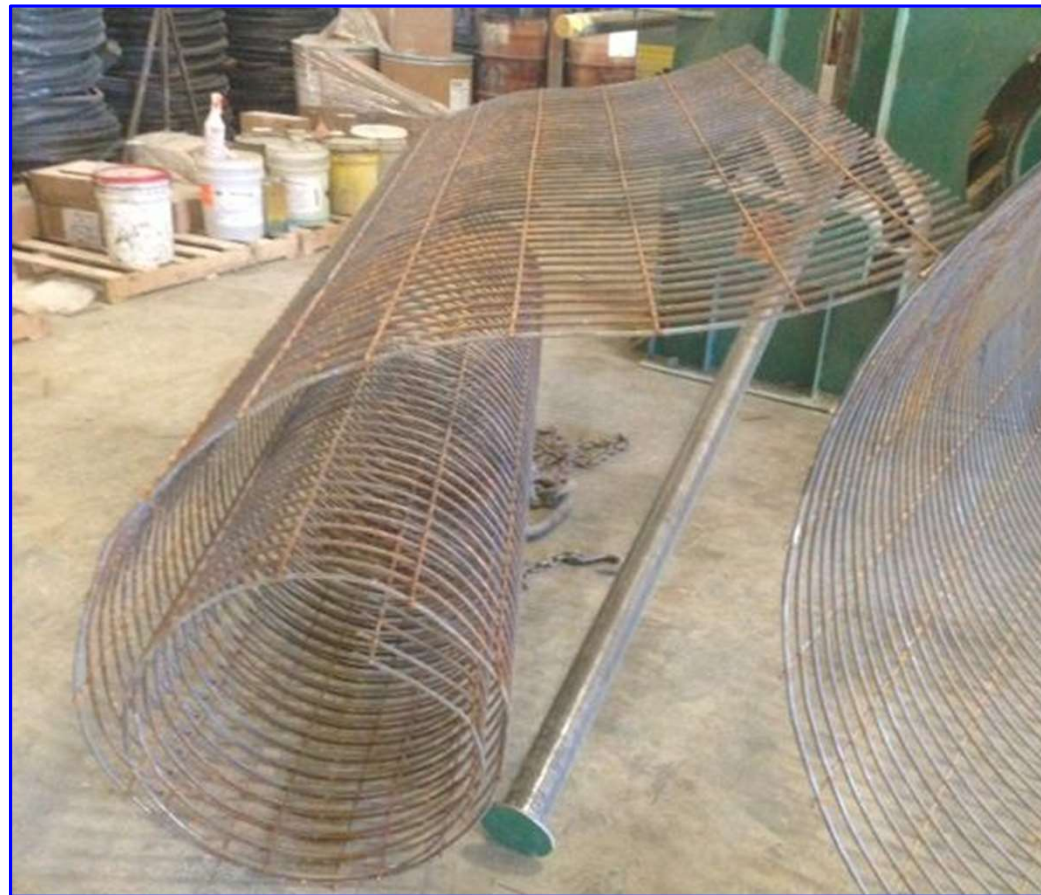
Improper Mesh Rolling Machine Set Up
