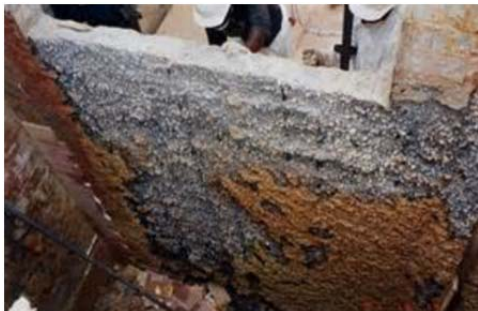
Fig. 8-10. Damage to concrete exposed to acidic environments.
