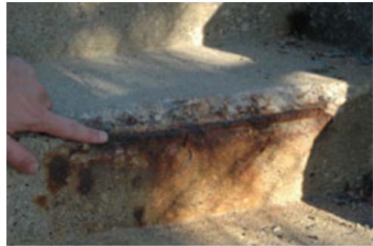
Fig. 8-12. Corrosion of steel embedded in concrete.
