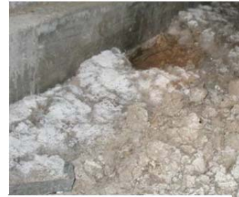
Fig. 8-9. Damage to concrete from soils containing salt.
