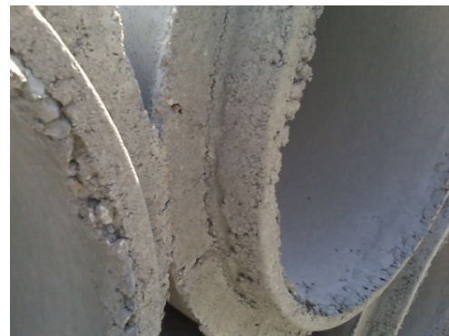
Fig. 1-5. Illustration of poor quality joints.
