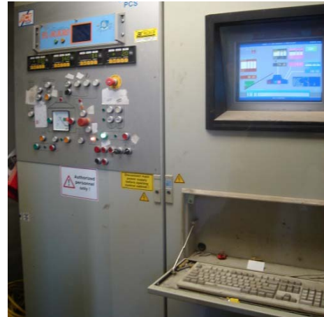
Fig. 2-1. Control room for batching equipment.
