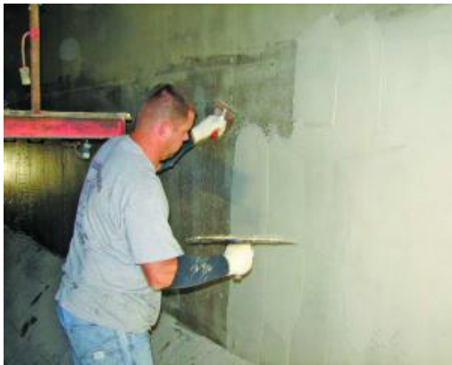
Fig. 2-9. Illustration showing epoxy mortar being applied due to cracking or material defects.
