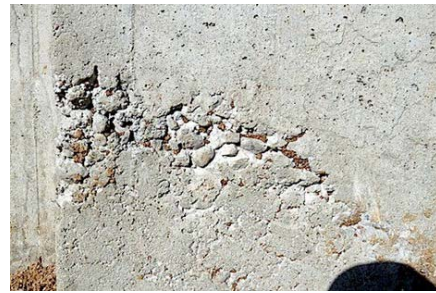
Figure 3-4. Illustration of honeycomb in finished concrete.
