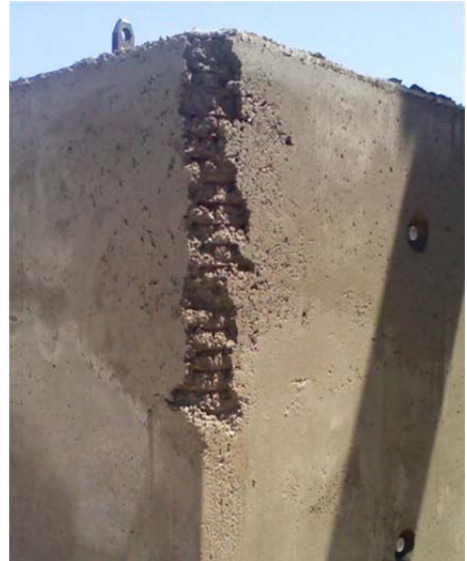
Fig. 3-1. Example of defects in concrete due to improper consolidation.
