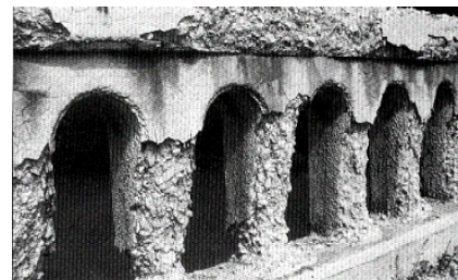
Fig. 8-3. Concrete deterioration due to freeze/thaw.
