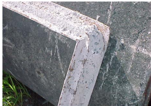
Fig 2-3. Example of a dirty joint ring.
