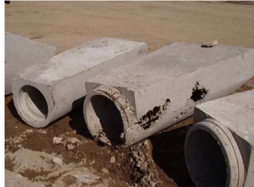
Fig. 1-4. Illustration of exposed steel found during a post-pour inspection.
