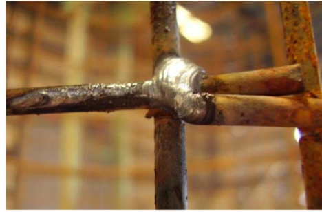
Fig 2-5. Example of a poor lap/ weld.
