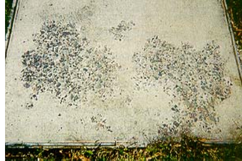
Fig. 5-7. Example of surface damage due to freezing and thawing.
