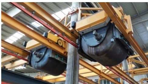
Fig. 2-13. Traveling bucket conveyor.
