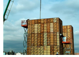
Fig. 7-12. Elevator shafts poured in a single lift using SCC, despite concern that the forms were not strong or tight enough to handle the pressure.
