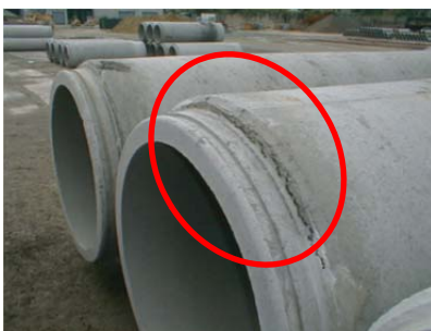
Fig. 2-3. Illustration of crack in pipe.
