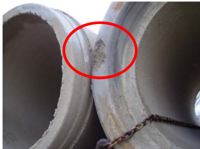
Fig. 2-2. Illustration of minor defect on top of older repair.
