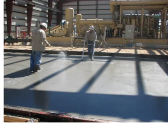
Fig. 7-11. Self leveling slabs require only minimal finishing to get a flat floor. Lafarge Agilia
