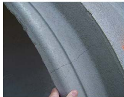
Fig. 1-8. Illustration of a crack in a spigot that extends all the way through and the entire depth of the joint; should be rejected.
