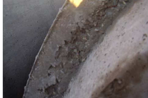
Fig. 2-7. Illustrating of the end of a bell, where concrete stuck to the pallet and pulled from the pipe, as a result of not having enough release agent.
