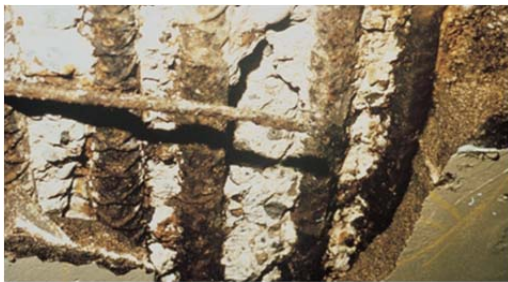
Fig. 5-6. Illustration of damage to concrete parking structure resulting from chloride-induced corrosion of steel reinforcement.
