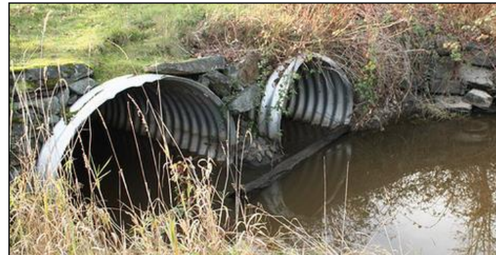
Improper Culvert for Cover/Backfill
