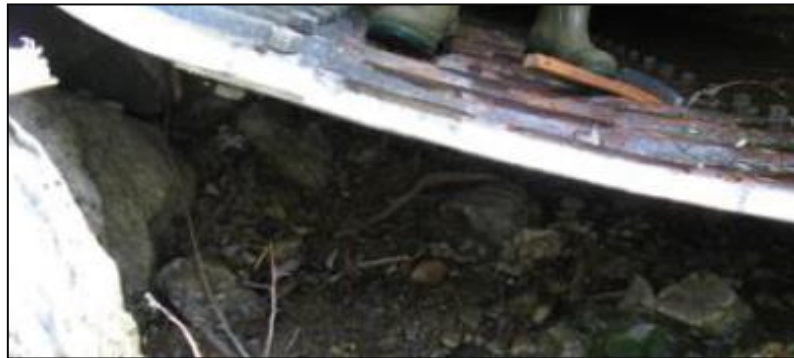
Undermining and Washout
