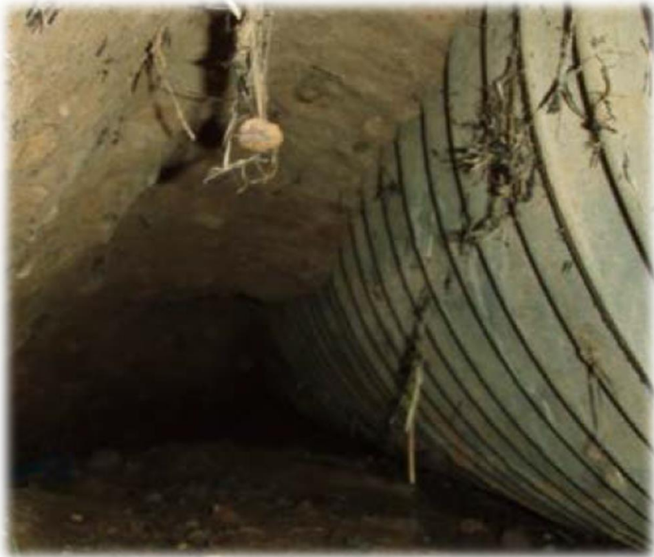
Loss of Soil Envelope
