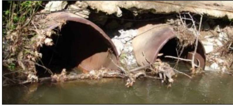
Increased Runoff from Development
