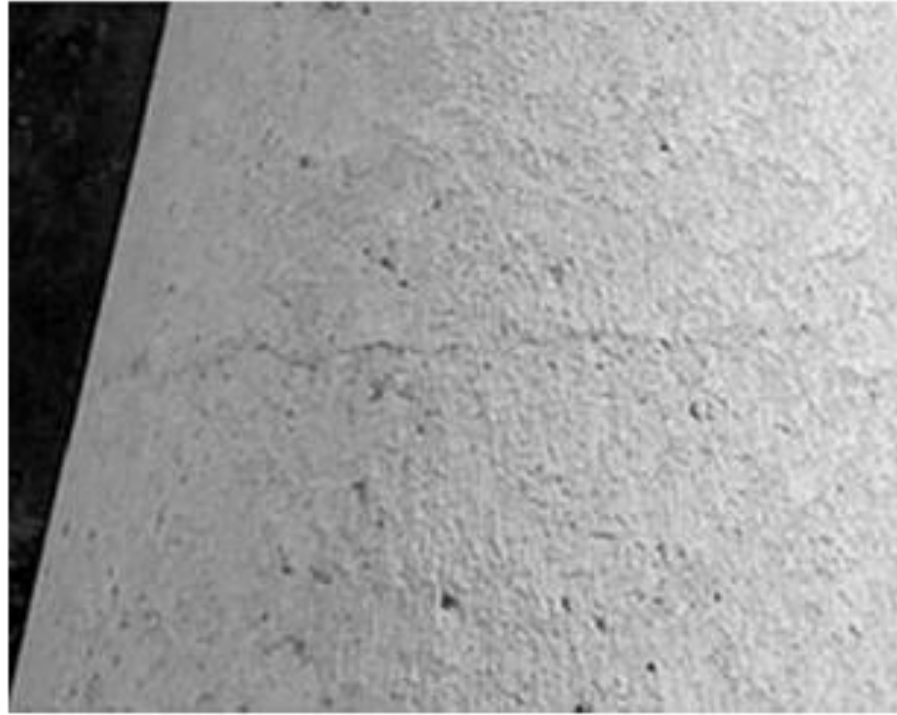
Figure 4—Acceptable Surface/Curing Crack (Photo Courtesy of ACPA)
