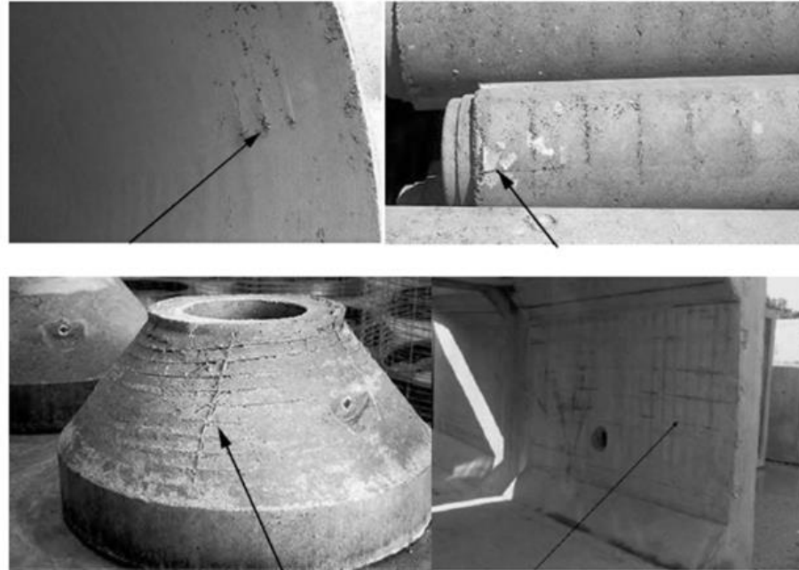
Figure 31—Rejectable Pipe, Conical Top, and Box Culvert with Exposed Reinforcement (Photo: Courtesy of ACPA)
