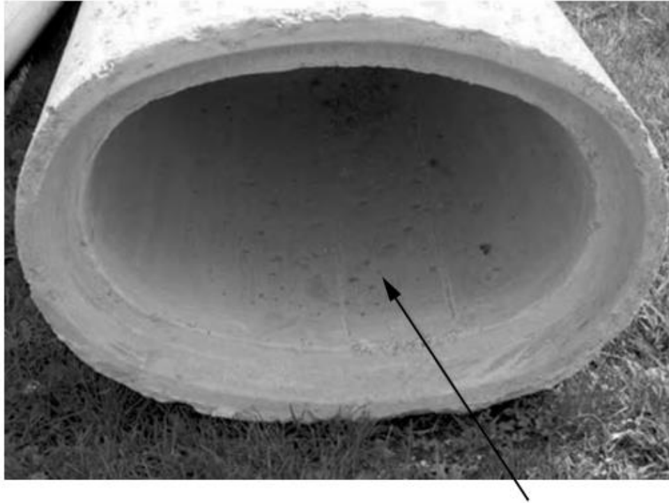
Figure 6 —Acceptable Bug Holes and Shallow Pitting (Photo Courtesy of ACPA)
