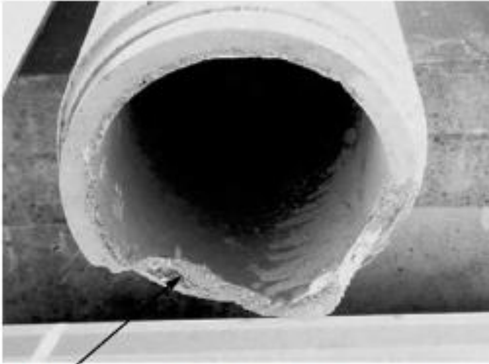
Figure 34—Rejectable Chipped and Damaged Spigot (Photo Courtesy of ACPA)
